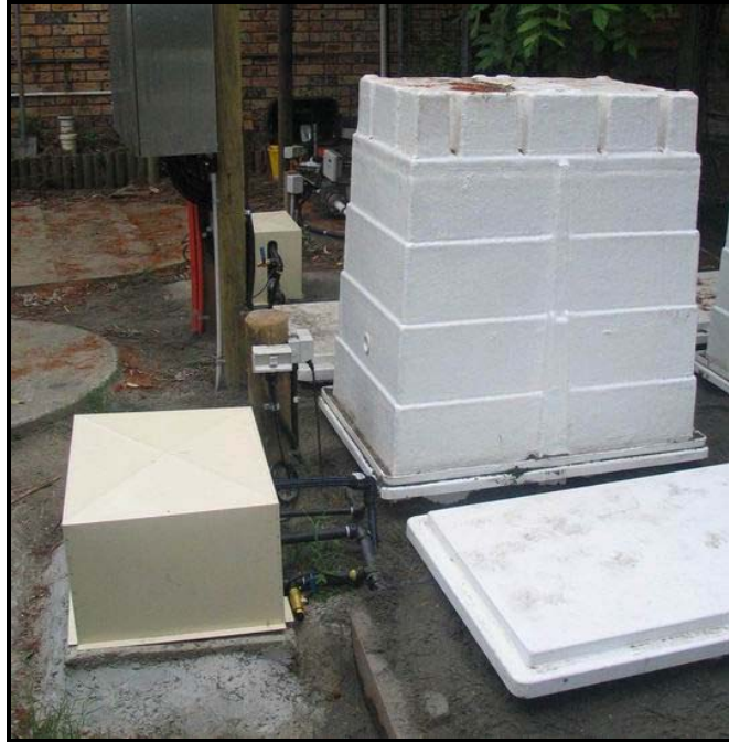
Figure 1: Caravan Park Test Site Installation
