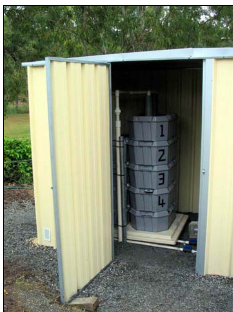
Figure 2.5: Tamborine, QLD Test Site Installation
