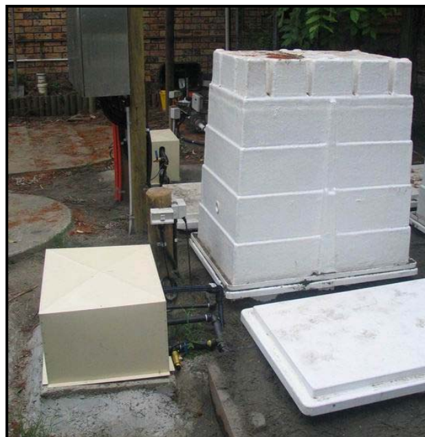
Figure 2.3: Caravan Park Test Site Installation
